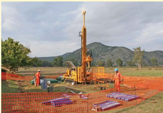
Fig.4: Fugro’s drilling rig on location at the southern Livadi Marsh, early October 2010.
